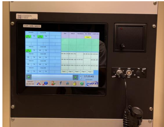
Figure 2 CWP: rack mount
